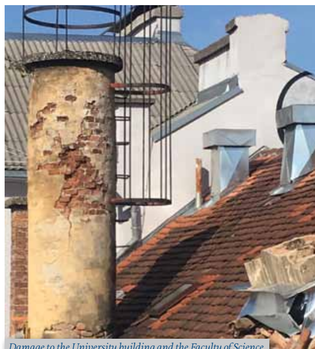
Damage to the University building and the Faculty of Science
